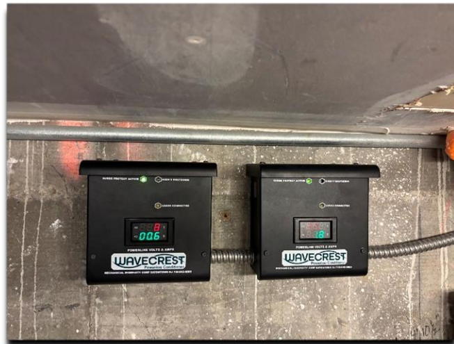
Figure 5: (2) of the 120v units installed in the wine cellar, down the stairs from the electrical panel that was in the hallway. Note: iPhone cameras have a hard time capturing the voltage readouts.
