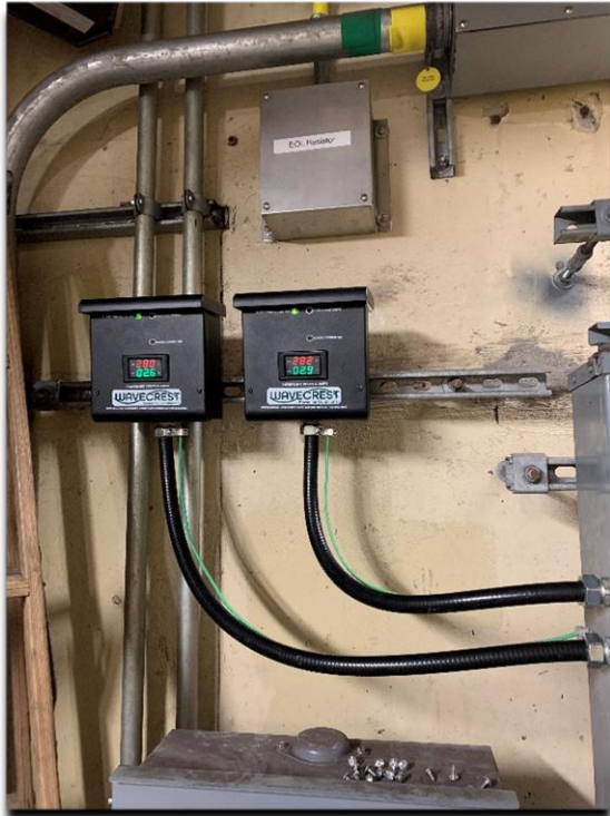
Figure 3: Wavecrest installed on 2 of the lighting circuits for the MTA
