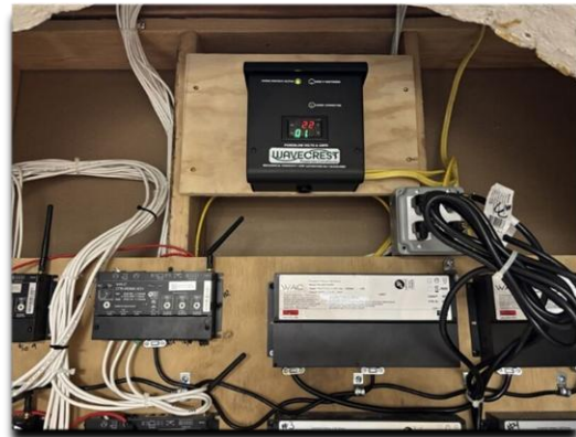
Figure 9: One Wavecrest stopped the problem in the whole house!
