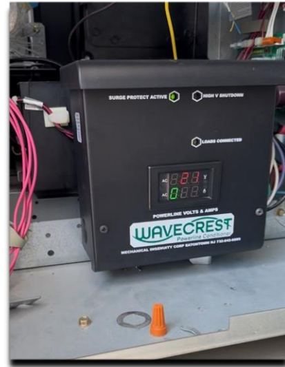
Figure 6: Initial sample installation at a particularly problematic pump. We encourage customers to try Wavecrest on the most troublesome circuits they have!
