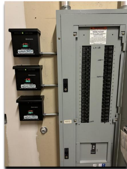
Figure 1: Wavecrest installed on each lighting circuit
